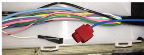
25. Insulate the cut end of the white wire and secure before closing the box.
