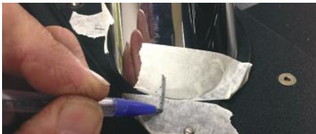
18. Use masking tape and a pen to mark the positions of the plates relative to the bar.
